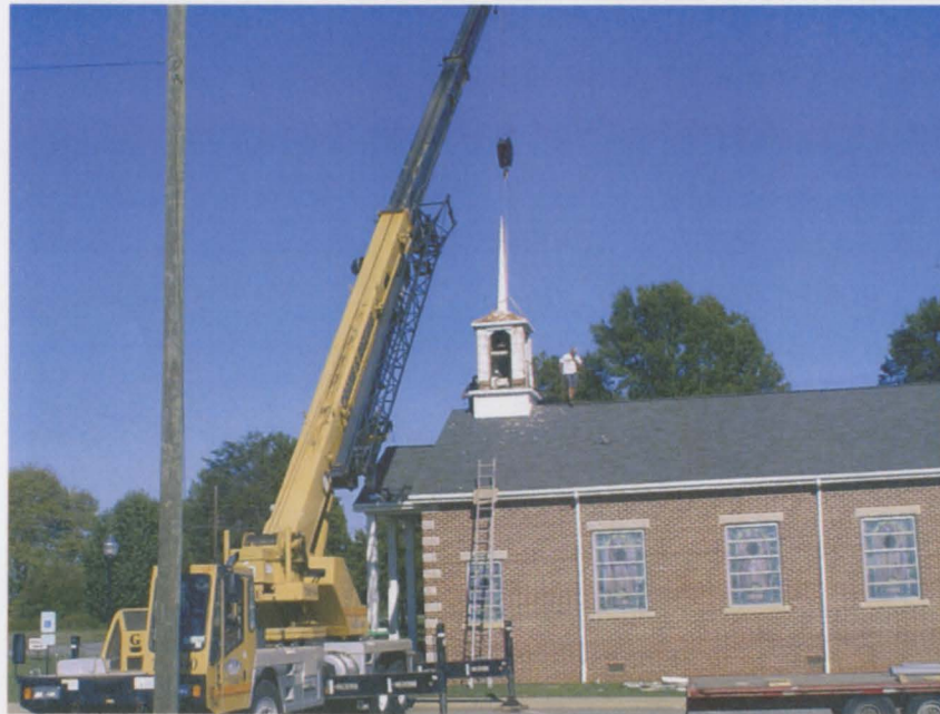
A crane prepares to lift Fairview's steeple from the building on October 10, 2007.
