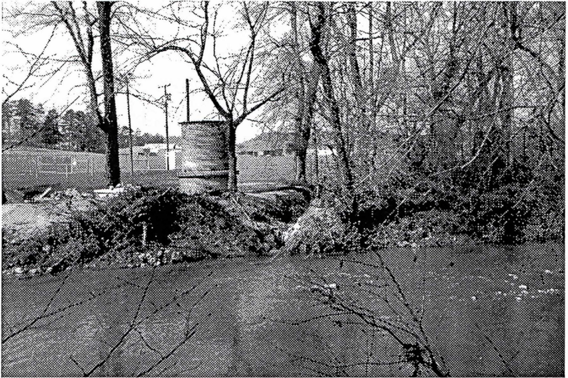
Veteran's Park Infiltration Pump Station
