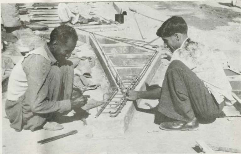
Making precast reinforced concrete beams for the roof of the domestic staff quarters of New United Christian Hospital.
