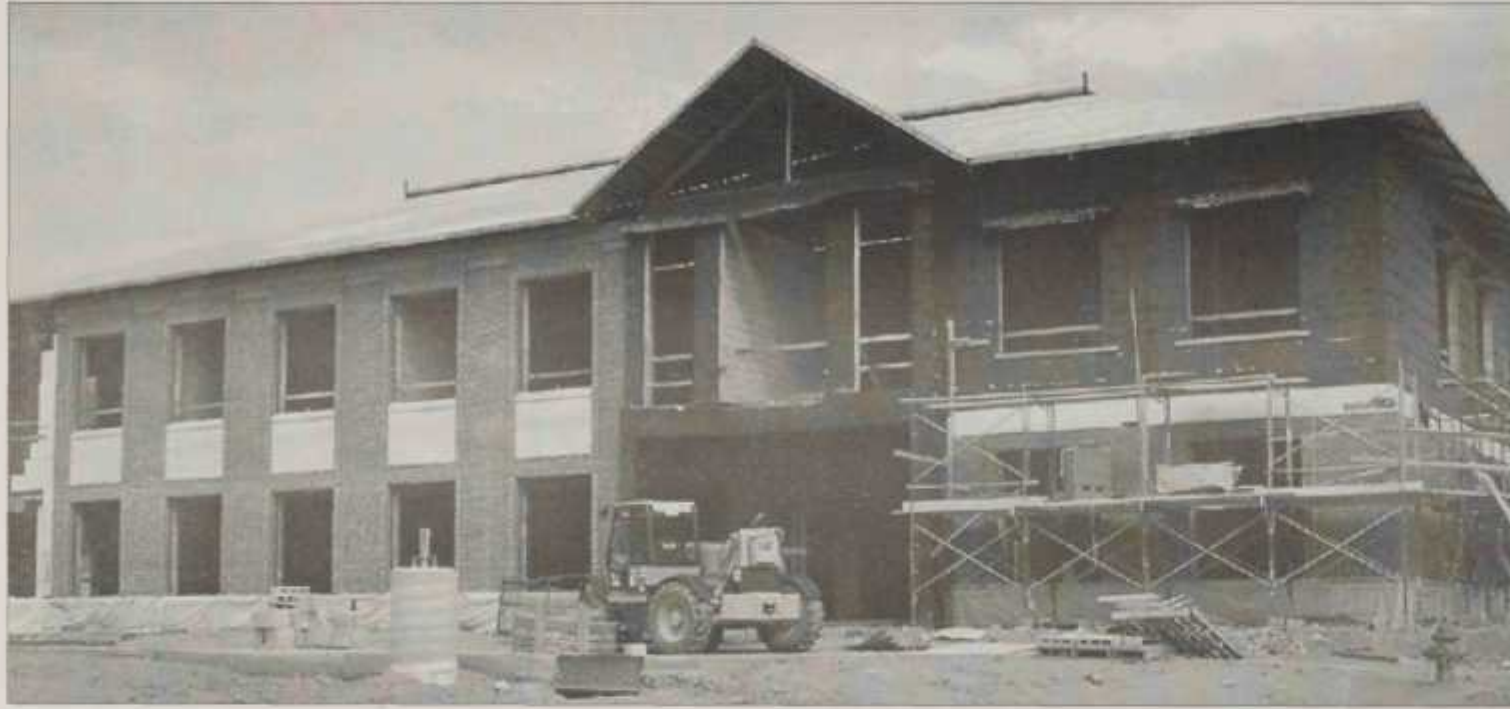
Drivers by can now see the building taking shape, serving as the northern gateway for Yadkinville.
