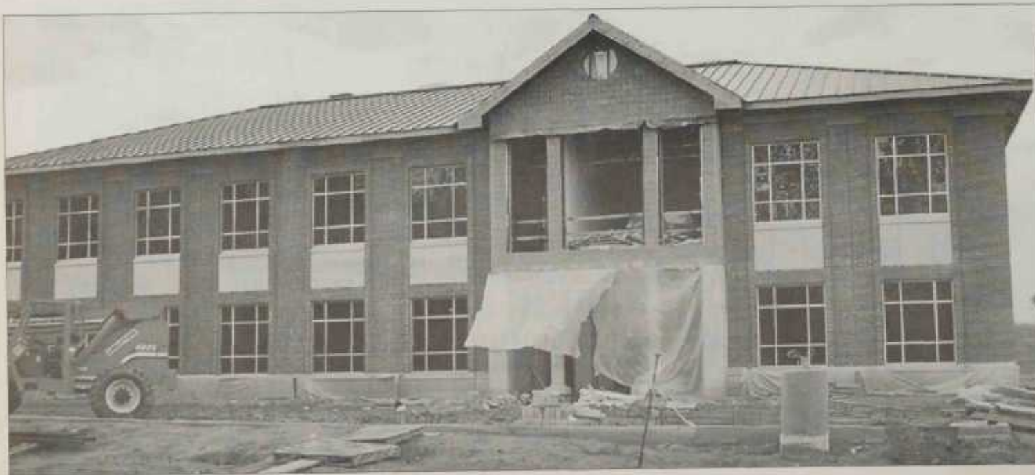
Windows now in place, workers prepare to landscape the grounds and wait for furniture to arrive.
