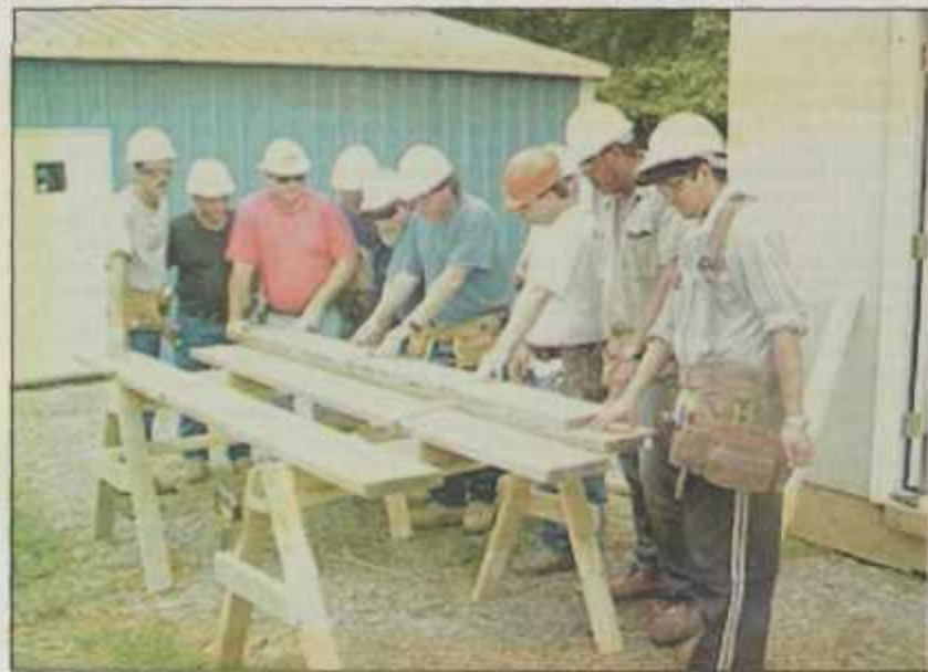
Instructor Joe Wilkins, third from right, works on a project with construction workers, from left, Charles Smith, Greg Hankeison, Kim Davis, Alvid Flores, Timmy Johnson, Pete Barr, John Parker, Gerald March and Alex Flores.
