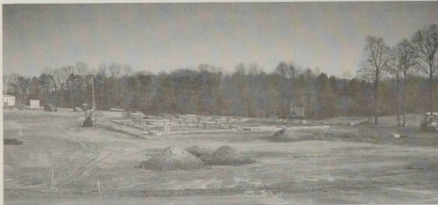
Workers begin to lay the foundation for the new Yadkin campus, which has been in the planning stages since 1996.
