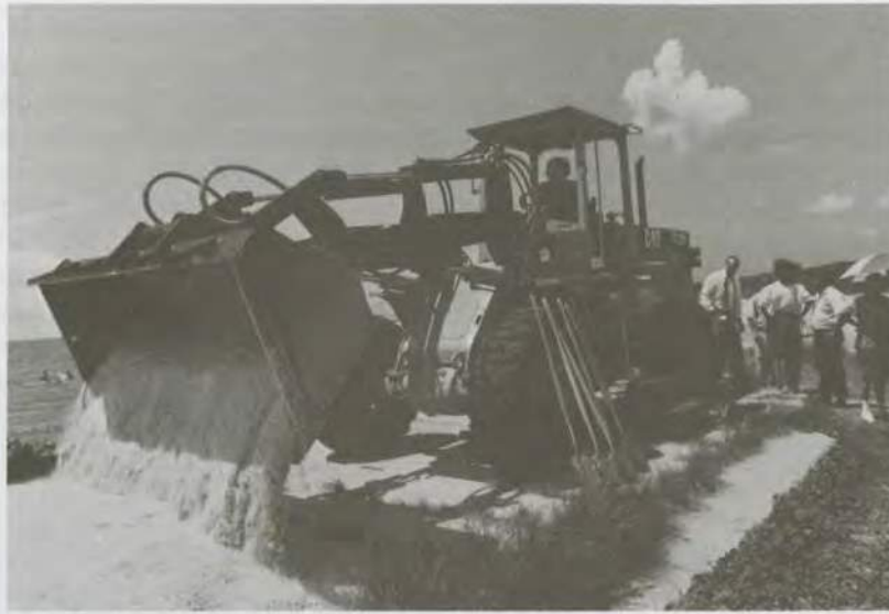
On July 15 Misener Marine Construction Company inaugurated efforts to construct a massive stone revetment to protect historic Fort Fisher from erosion by the Atlantic Ocean. During special ground-breaking ceremonies attended by a number of state officials, Secretary of Cultural Resources Betty Ray McCain dumped the first load of dirt from a front-end loader.
