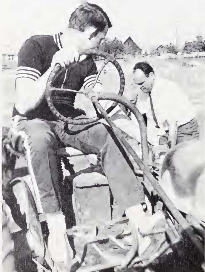
Coach Doug Cook stopped the tractor as Mr. Wilburn and Mr. Donnell adjusted equipment for grading new baseball field as season began.
