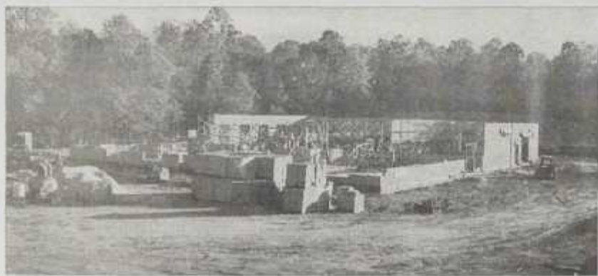
Construction moves forward as John S. Clark of Mount Airy, the general contractor, moves more dirt and lays the brick for the college's first new building outside Surry County.
