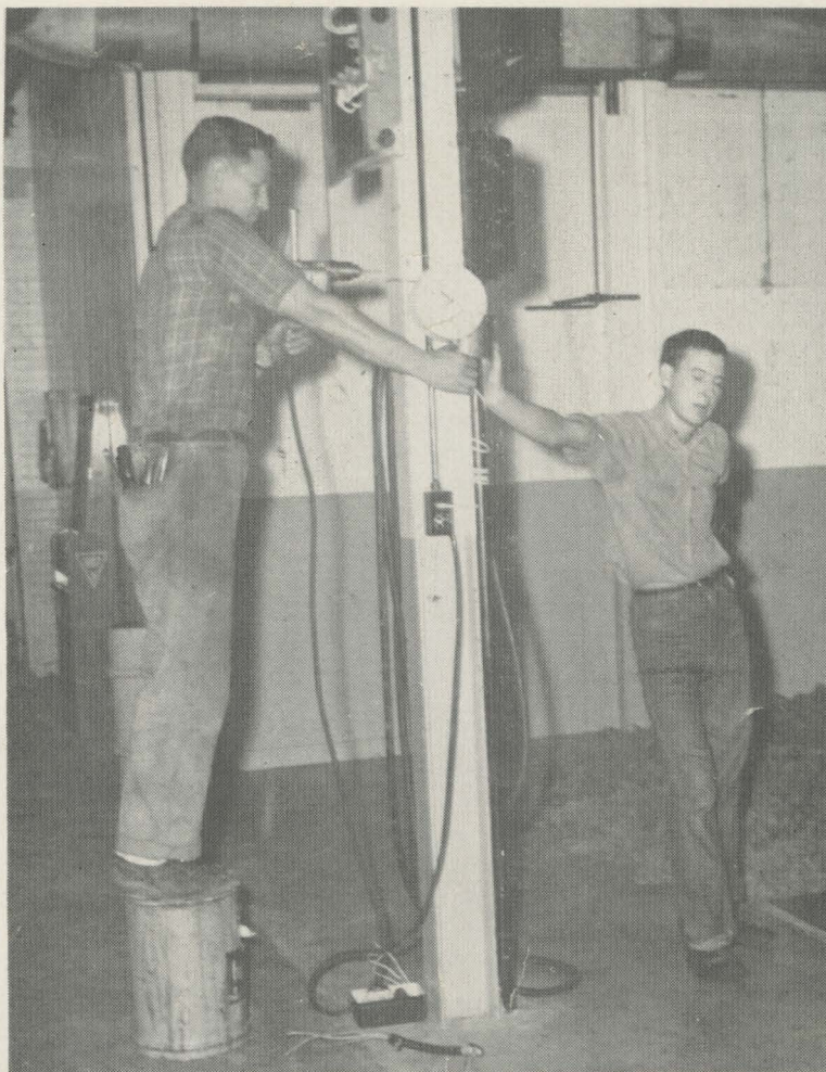
CHARLES HARRIS of the Electrical Department is drilling for some electrical installation, while Buster Luffman, with eyes closed accidentally, is pushing a switch button to start his machine. (Staff Photo)
