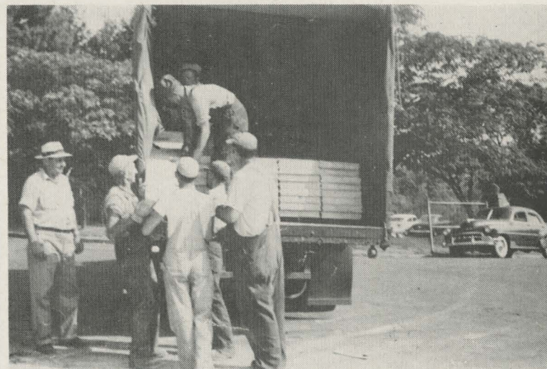
WALTER BARNETTE, left, and Herman Hinson, contracting foreman, extreme right, are shown with a group of hefty fellows unloading concrete "decking" for the roof of an addition to the Piece Dyeing department. (Staff Photo)
