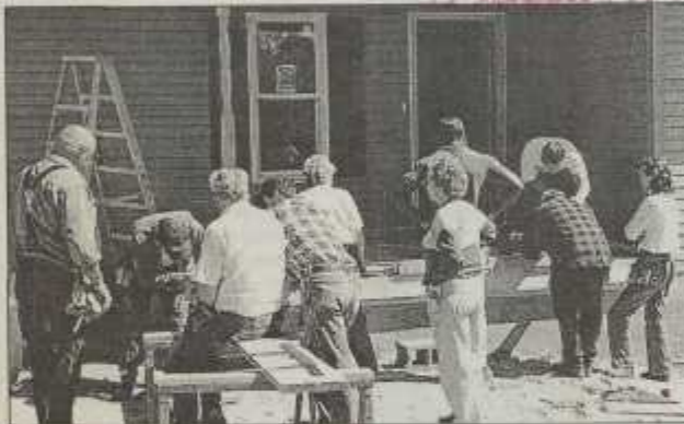
COMPLETING THE PORCH —Surry Community College students put the final finishes on the porch at the house of Craig and Lisa Smith of Robin Road, Boonville. Pictured are (l-r): Bruce Bowman, Patrick Inman, Leon Hayden, Andy Collins, Susan Sutphin, Eloise Stinson, Danny Gist, Henry Johnson, Chris Allen and Sabrina Nixon. (Lynn Templeton-Photo)
