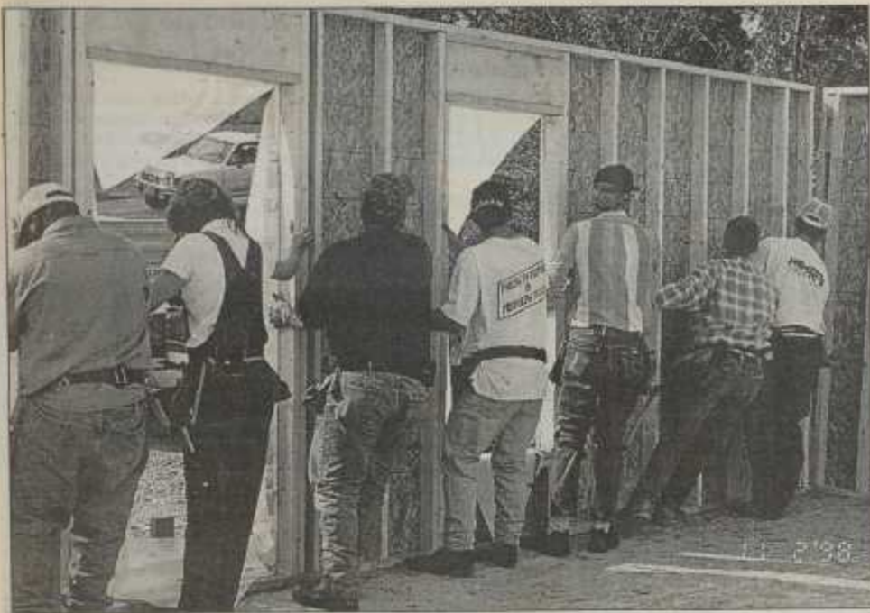
A WALL GOES UP —Students from Surry Community College install one of the walls of the Craig and Lisa Smith house, located at 105 Robin Street in Boonville. In the photo, which was
