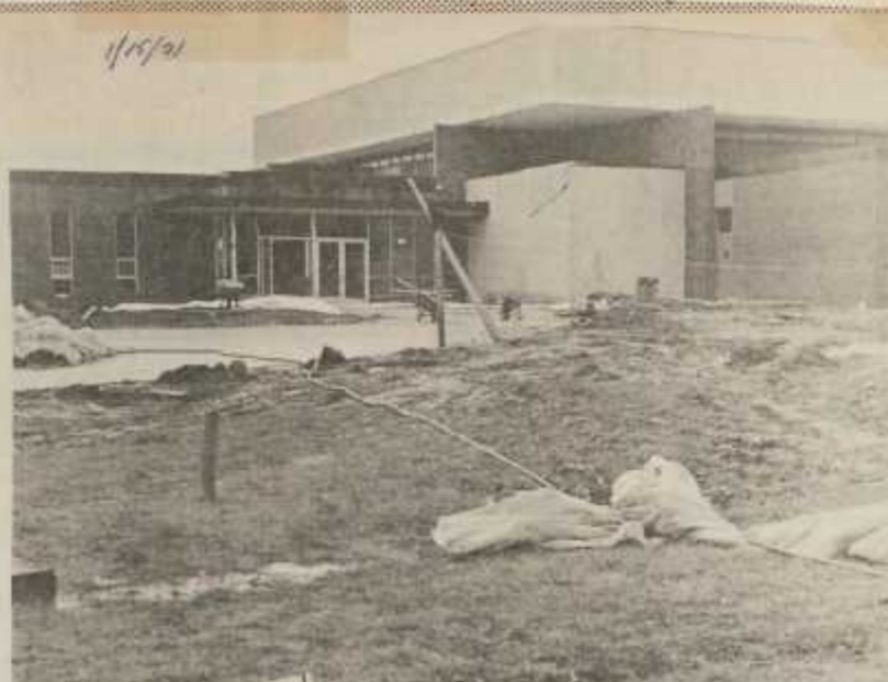
The new Surry Community College Gym is nearing completion. (Tribune Photo by Rebel Good)
