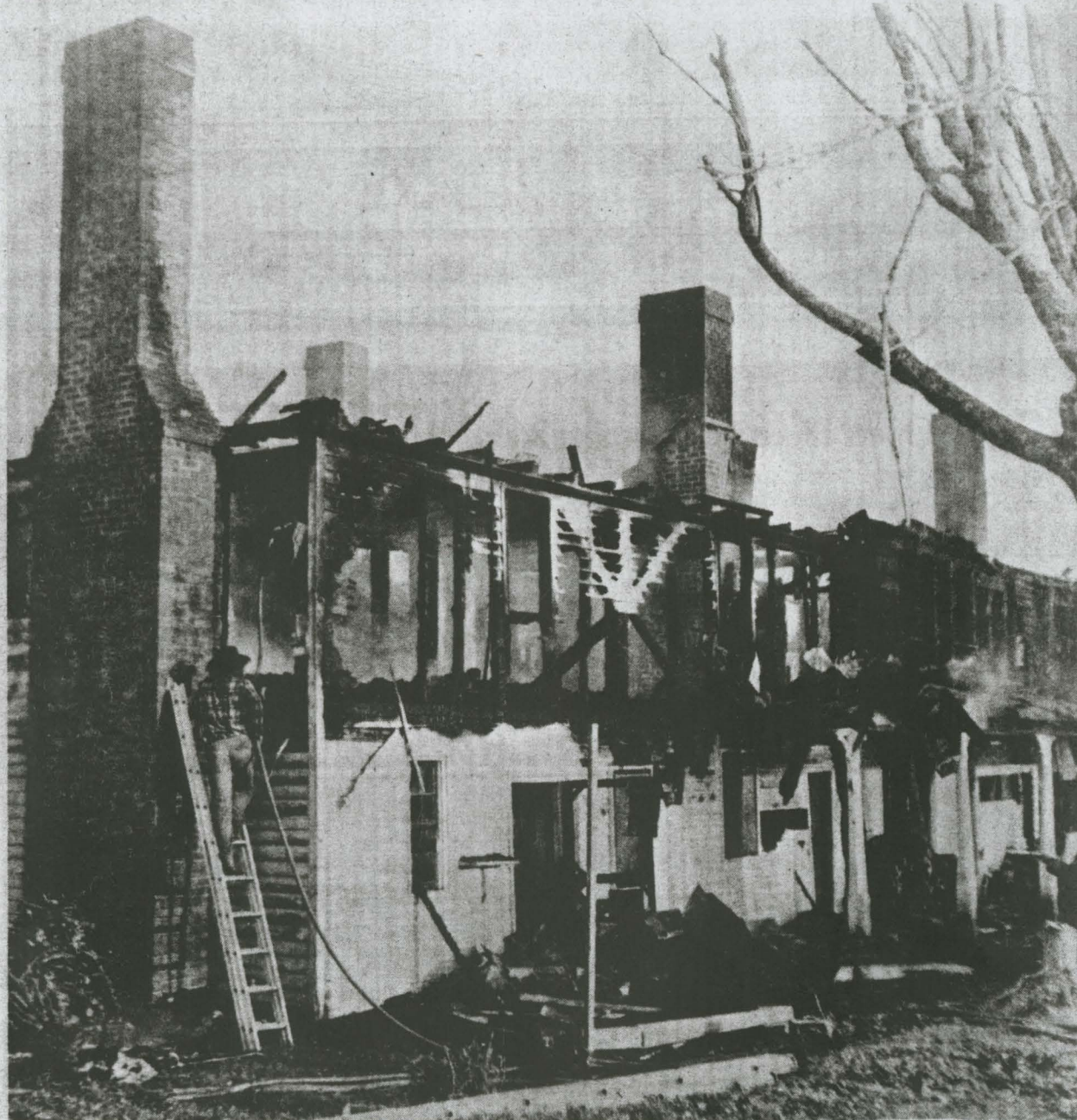
Randall Agee assists firemen in the effort to extinguish the smoldering walls and floors of the Grant-Burrus Hotel.
