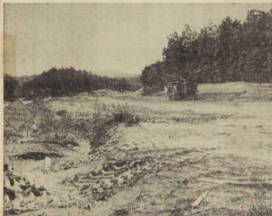
Grading work on new U. S. Highway 601 moved steadily closer to Mount Airy this week. This picture was snapped Tuesday afternoon near the Franklin Road-601 intersection, and some embankment work had already progressed further in this direction. Work on the Highway 601 project began in early June and is expected to be completed by next fall. (TIMES Photo)
