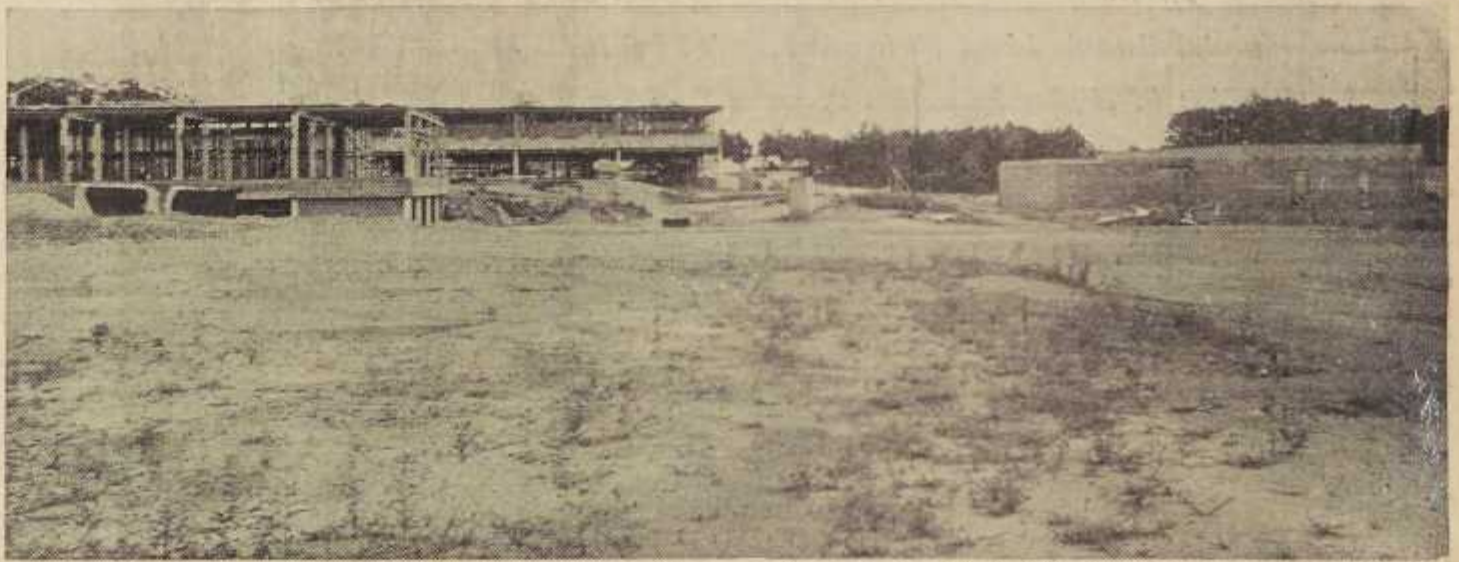
The construction site at Surry Community College, showing all three buildings. They are, from left, learning resources, science-technology and shop. Construction, according to I. John Krepick, college president, should be about one-third completed, but is lagging behind schedule. Target date for completion of the first three structures is spring, 1967.
