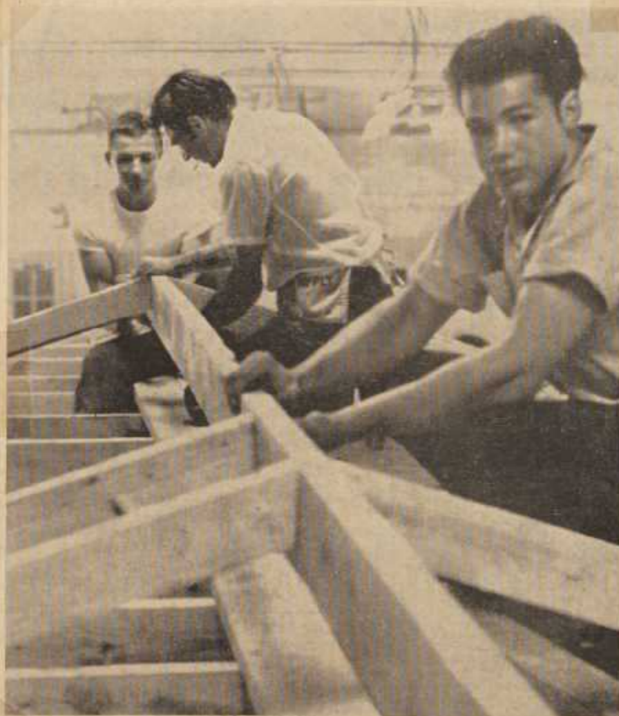
...Wade Haynes, Jimmy Potts and Arthur Wilson (l-r) help build a house within a house... —NEWS Photo
