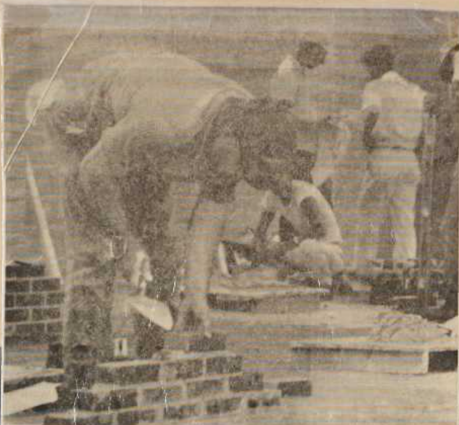
NEW HOPE FOR THE FUTURE is expressed by the hands of this student as he practices the techniques of laying brick at the classes now underway in Mount Airy. Sponsored and taught by Surry Community College, the federally financed program is in the process of training apprentice bricklayers to a degree of proficiency to enable them to leave the classroom and begin on-the-job earnings immediately upon graduation. MT Airy News June 21, 1966 —NEWS Photo
