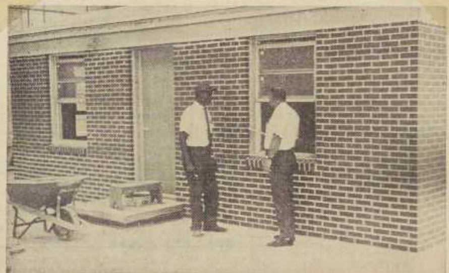
LEVI S. GEE, SURRY COMMUNITY COLLEGE MASONRY INSTRUCTOR, and George Jones, carpentry instructor at the college, look over the exterior of the newly-completed house their classes have built in the old Town Tire building on the corner of Virginia and Willow Streets. When the house is completed, it will be torn down to make way for more projects of the classes, financed by a Manpower Development and Training grant and sponsored by the local college.
