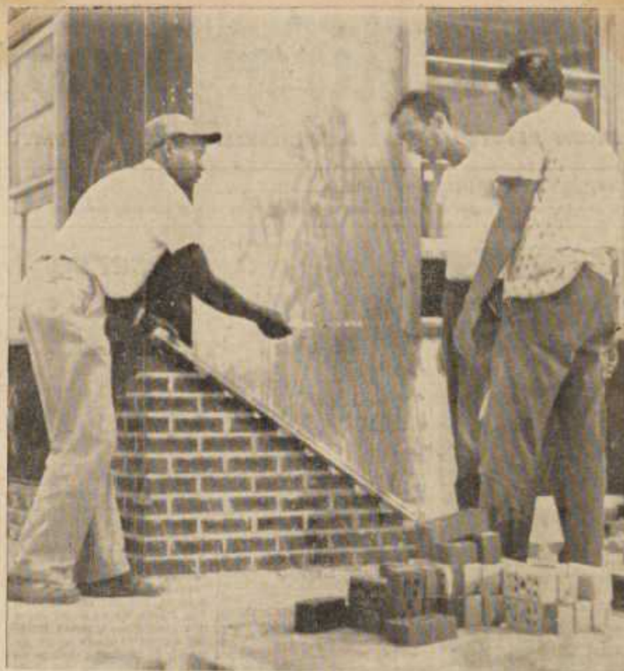
HOUSE-IN-A-HOUSE is getting a brick casing. Instructor Levi S. Gee, Jr., (left) instructs Richard Young of Fancy Gap Road and John A. Carrico of Reeves Drive into the proper techniques of the most difficult part—the corner. The work is part of the current class of bricklaying instructions held daily in the old Town Tire Building at Virginia and Willow Streets. The courses are under the extension department of Surry Community College. Jimmy Reeves serves as coordinator. All techniques of a real house are followed on the pictured project, except that lime mortar is used for easier tear-down when it's finished. (NEWS Photo)
