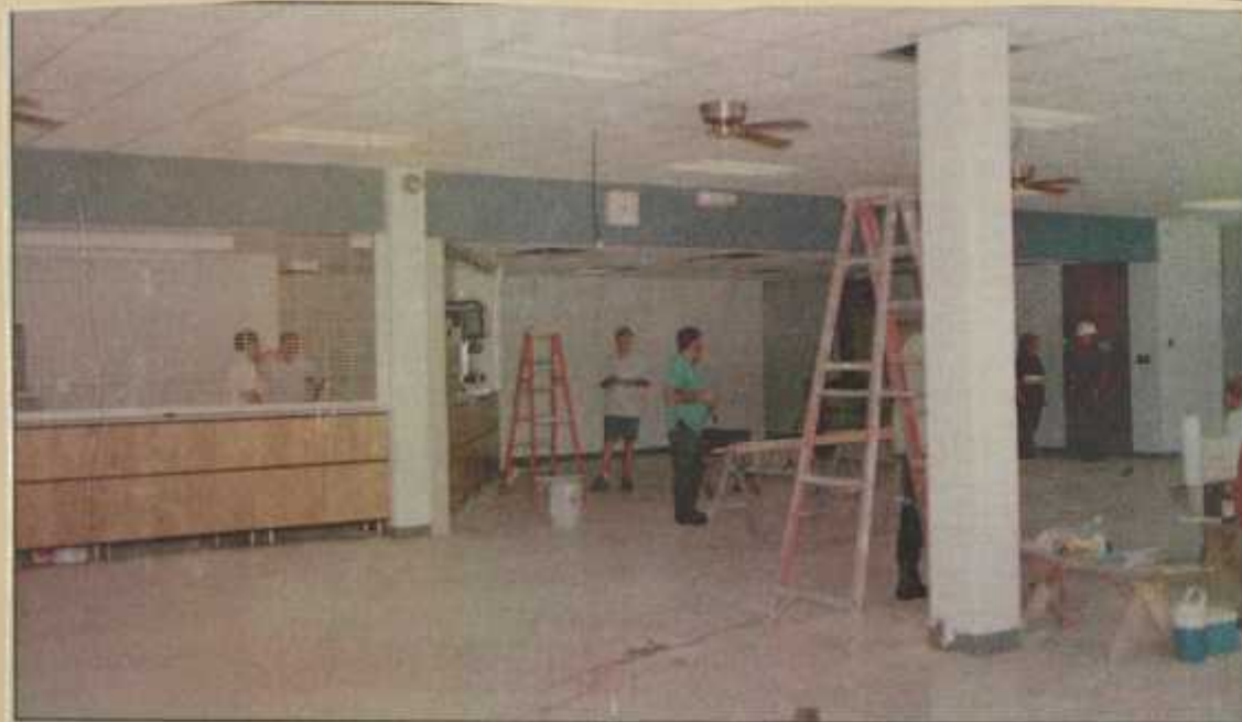
NEARLY COMPLETE: Electricians handle final wiring details while other workers take a mid-afternoon break Wednesday in the remodeled cafeteria at Surry Community College. The project is part of recently funded renovations to better meet student needs at the college.
